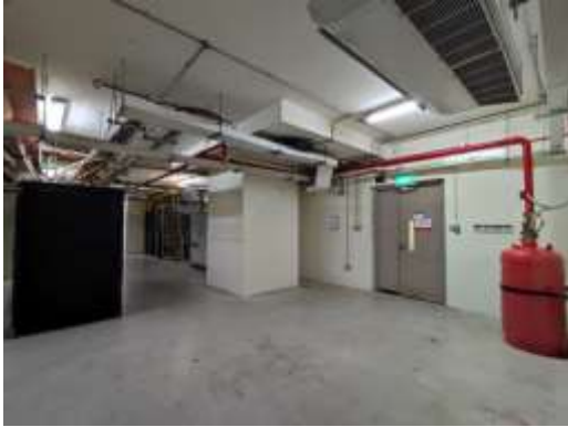
Gas Suppression System
