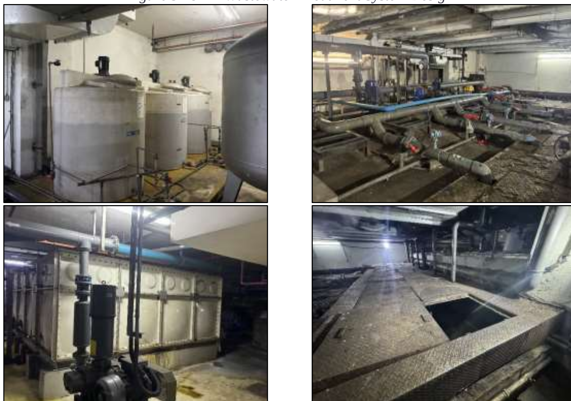
Figure 3-30 Current Equipped Wastewater Treatment System
